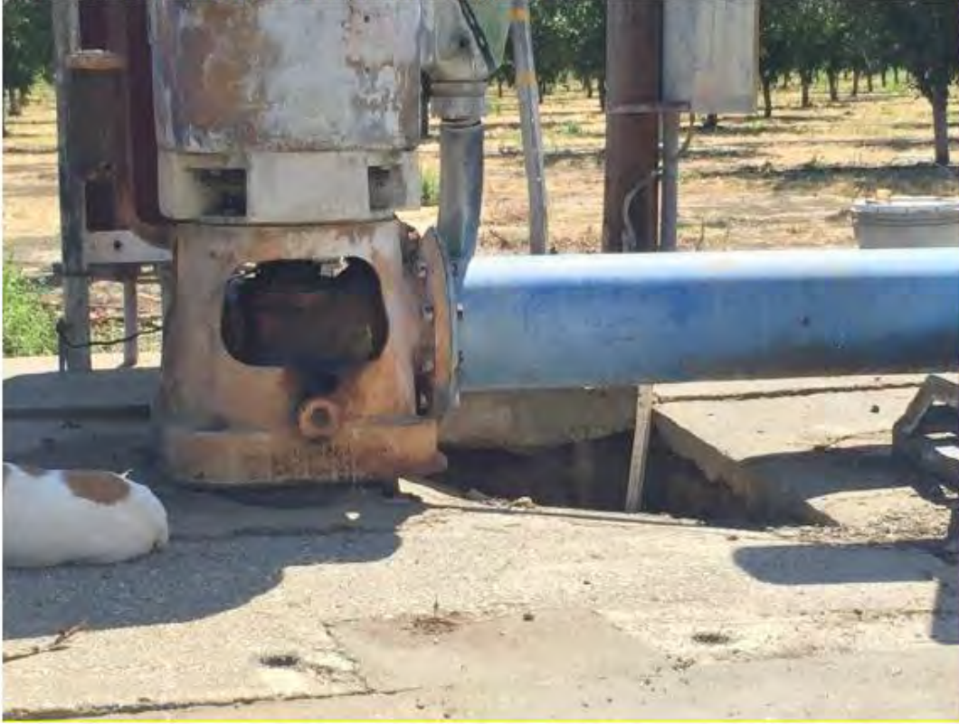
Figure 4. Subsidence on Billiou Well #35 pad. June 2015 (by Billiou).
